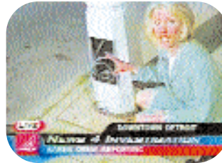
Exposing dangerous electrical wires on light poles near Detroit schools and playgrounds. WDIV / Detroit, July 19
